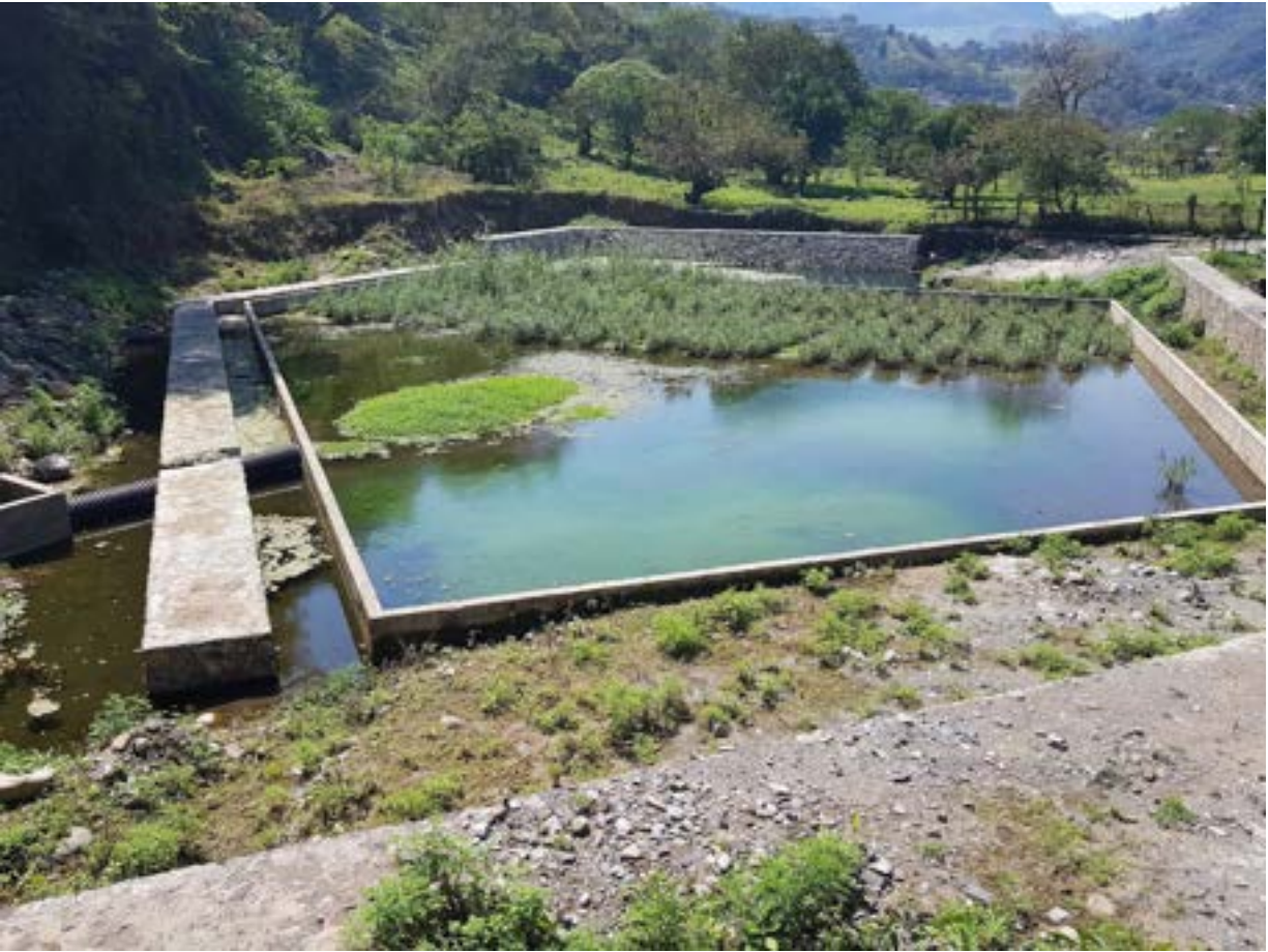
Wastewater treatment plant in Huehuetla. The wastewater treatment plant is a nature-based sanitation solution of wetlands
